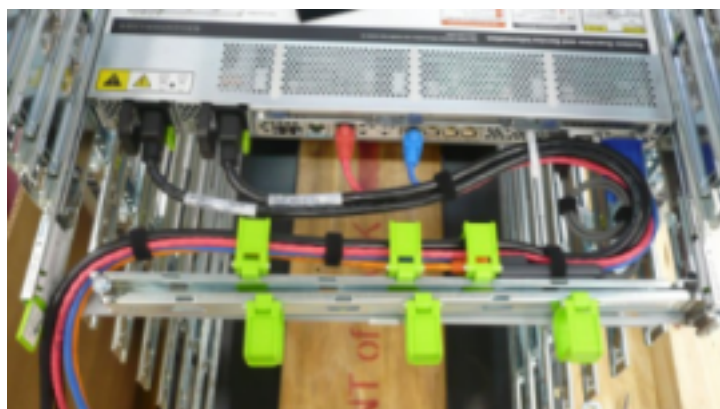
Figure 2-6 Cables Secured under the Cable Clasps
