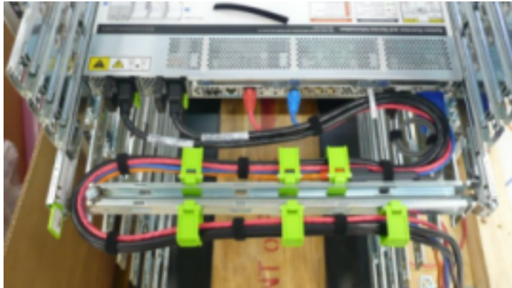
Figure 2-7 Cables Secured with Hook and Loop Straps at Regular Intervals
