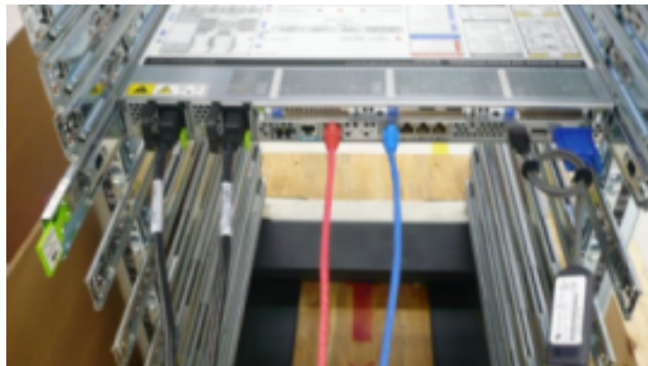
Figure 2-3 Cables at the Rear of the Server
