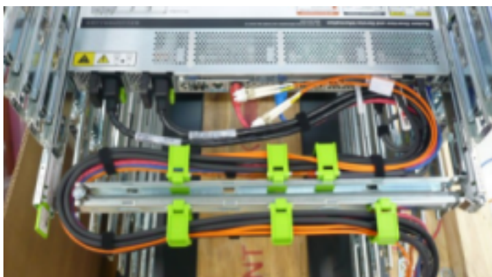
Figure 2-9 RDMA Network Fabric or TwinAx Cables Secured with Hook and Loop Straps at Regular Intervals
